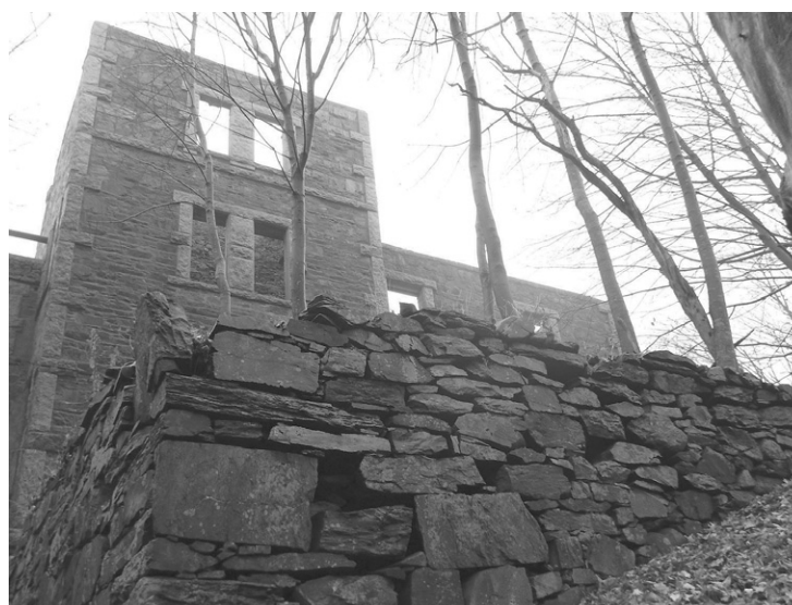
The Goddard mansion on a foggy Dec. 3. The Town Council, on Nov. 4, unanimously adopted a policy to continue stabilization of the mansion, reflecting views of the majority of citizens responding to a survey question on the subject.
